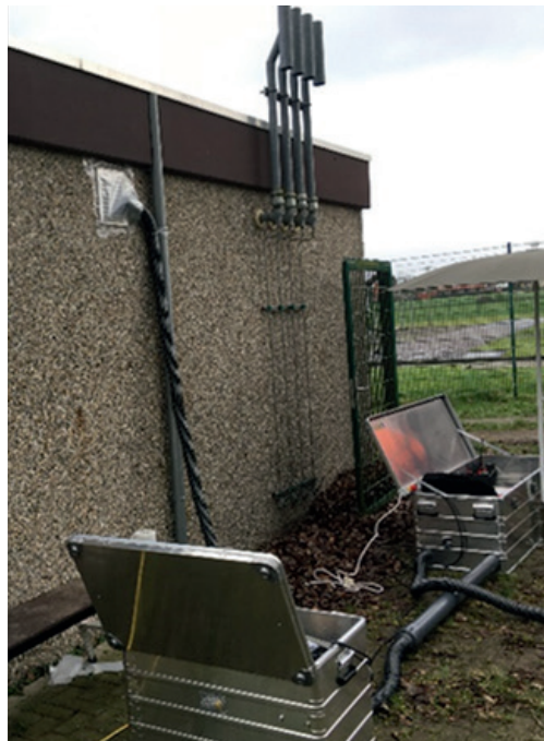
Figure 3 (left): Measurement Using the Suction Method at a Gas Pressure Regulating and Metering Station
